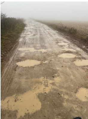
Image shows a compacted gravel path with puddles.
